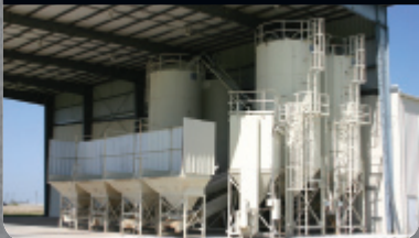
VINCE HAGAN BATCH PLANT
