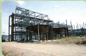
*Ethanol Plant Sits on 4.98± Acres Leased Land (City of Burley-Owner)
