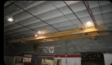
Two 2-Ton Bridge Cranes
